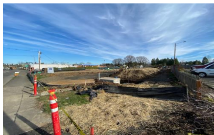
Hwy 213 at 211 is the future site of the Colima Apartments, a 36 unit complex.
