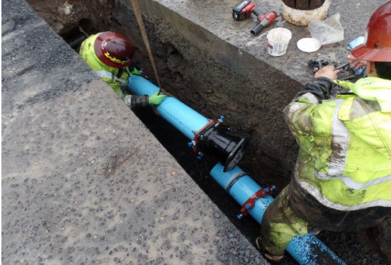
A New Water Main is Installed in the 500 block of W Main St. – Water loss was reduced by 15% this Fiscal Year!
