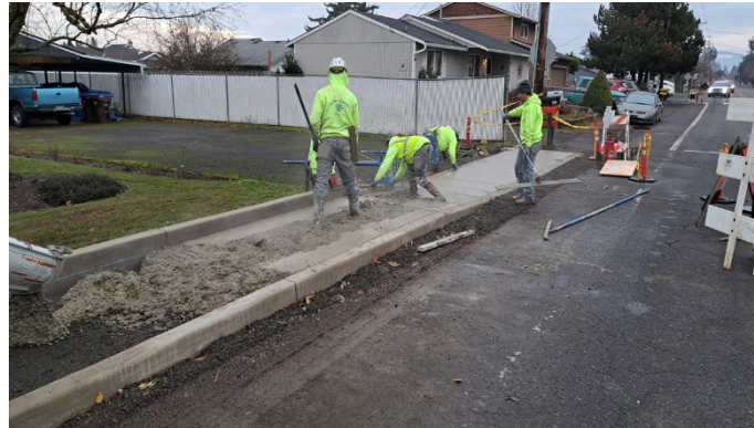
Sidewalk Infill in conjunction with an Emergency Water Main Repair on Toliver at N Leroy Ave
