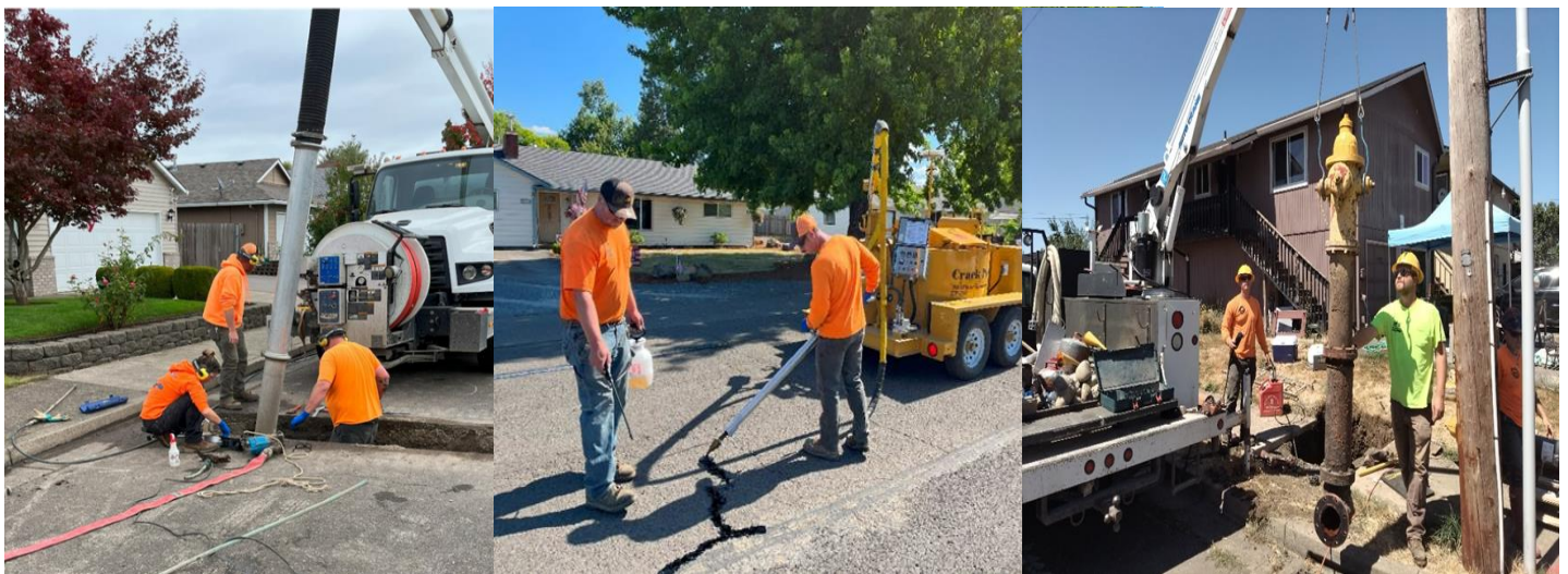
L: Using the Vac Truck while replacing a leaking water service line. M: Crack sealing is performed annually to preserve pavement as long as possible. R: Testing and (if needed) replacing fire hydrants is another ongoing job for the crew.
