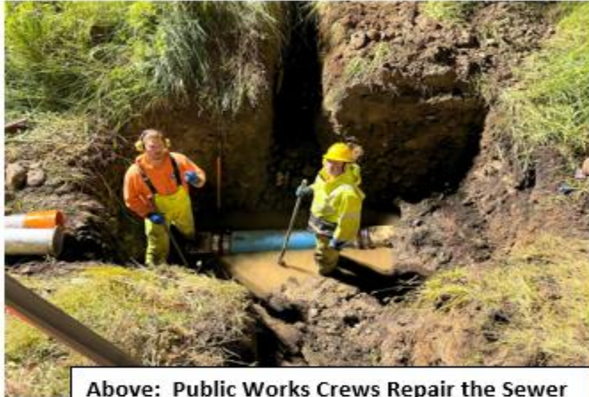
Above: Public Works Crews Repair the Sewer Main that was Damaged in the Roundabout Project.
