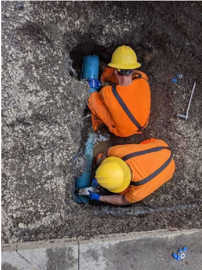
City Crews are constantly replacing and repairing water services and mains. Left, two new service saddles are placed on an 8" PVC pipe in Big Meadow, replacing more corroding copper services. Below, Devin unwinds new PEX Pipe for these new services, and Rich tightens steel bands on an older leaking mainline in July.
