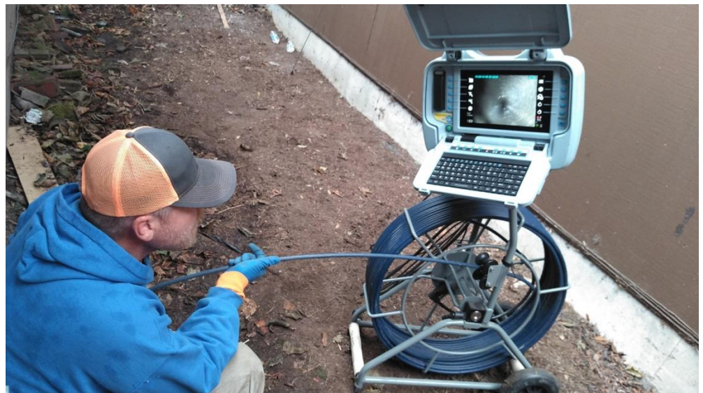
Right, Rich feeds the sewer camera into a lateral for a customer with a sewer backup. The City is responsible for sewer lines from the Property Line Cleanouts to the Main lines.
