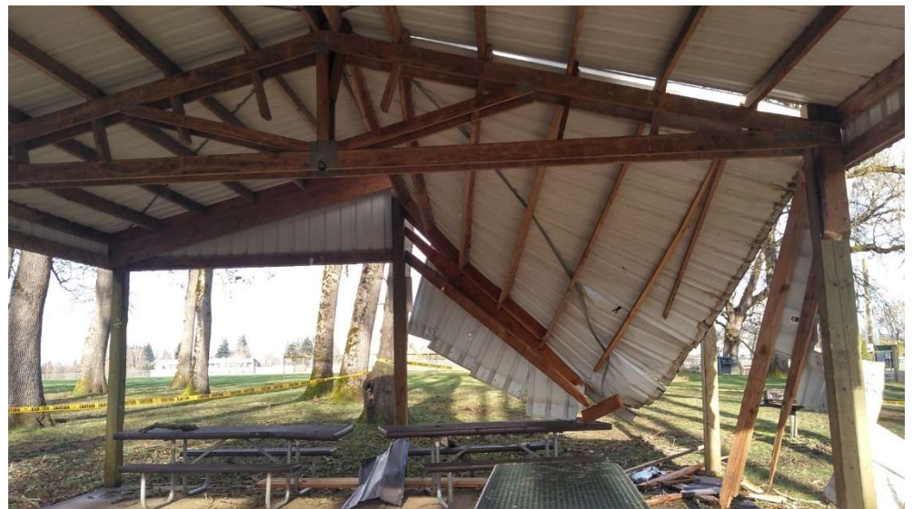
Right, Clark Park Pavilion was assessed for damages by the City's insurance provider. A contractor has been released to make the structure safe until further plans for the site can be made. A local Business, Interfor, has expressed interest in helping the City with donations. Staff will work with them once a plan can be approved.
