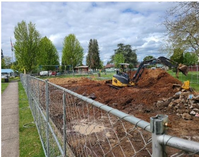
Left: Construction Crews Demo the Old Playground Equipment and Prepare the Site for its Fresh Equipment Upgrades.
