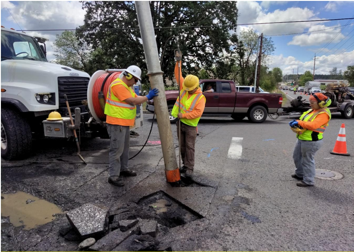
Above: City crew potholing water main for design of the Toliver roundabout.
