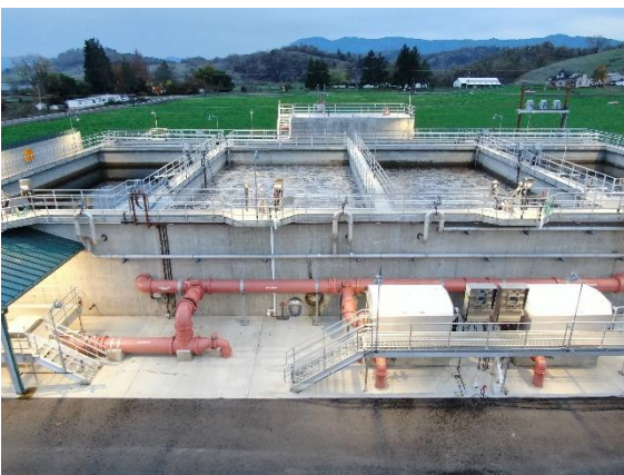
An example of the SBR type Wastewater Treatment Plant that will be built in Molalla, in part with Sewer SDC's
