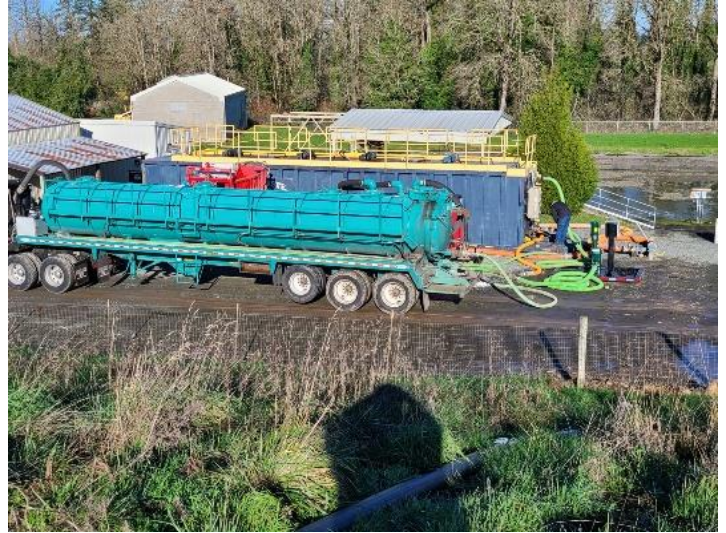
Biosolids Removal is now a continuous operation at Molalla's Wastewater Treatment Plant
