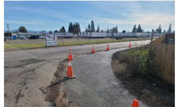
A new turning radius for Shaver Street removes a large systemic hole in the road.
