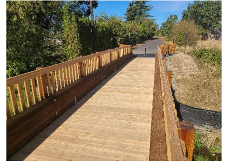
Looking North to Phase 3 of the Molalla Forest Road Project... Phase 2 brought this bike/ped bridge
