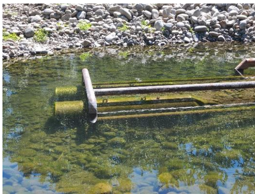
Molalla Water Intakes partially out of water - Summer 2021
