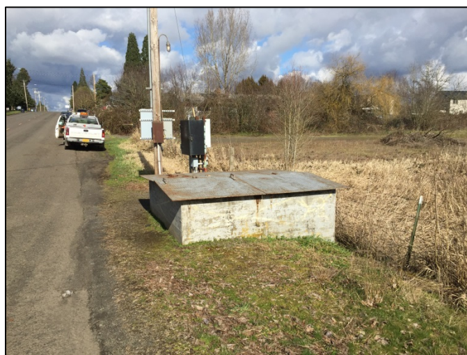
FIGURE 2.3.7 SOUTH MOLALLA PUMP STATION
