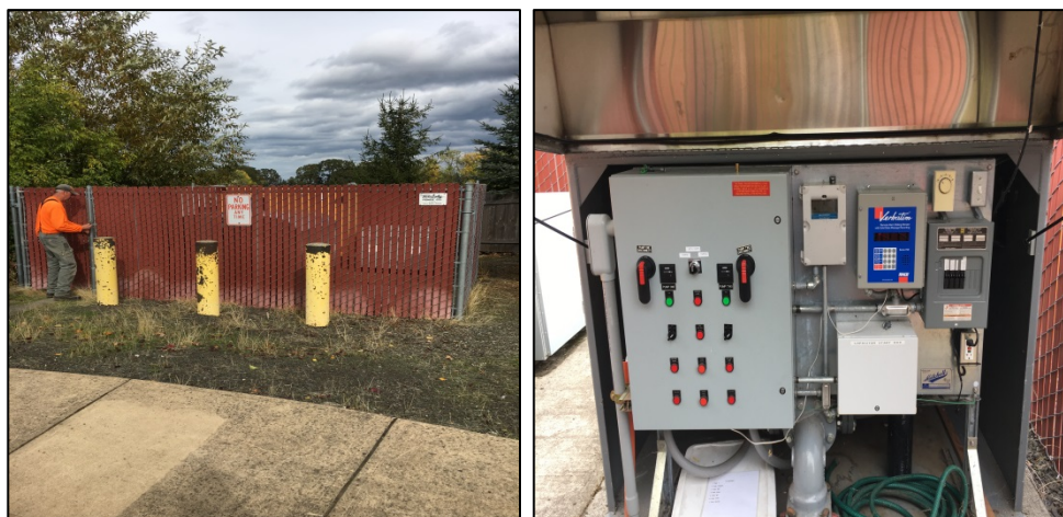
FIGURE 2.3.8 STEELHEAD AND COHO PUMP STATION
