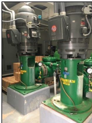
FIGURE 2.3.27 EFFLUENT PUMP STATION
