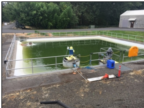
FIGURE 2.3.26 CHLORINE CONTACT BASIN
