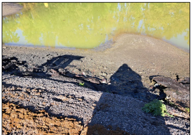
FIGURE 1 AERATION BASIN LINER FAILURE
