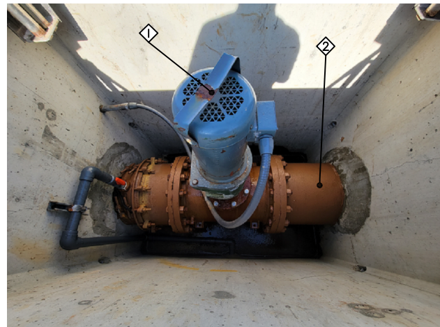
PHOTO: CHLORINE INJECTION VAULT
