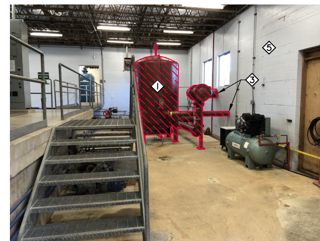
PHOTO: EXISTING DAF UNITS 6 100-D-8
