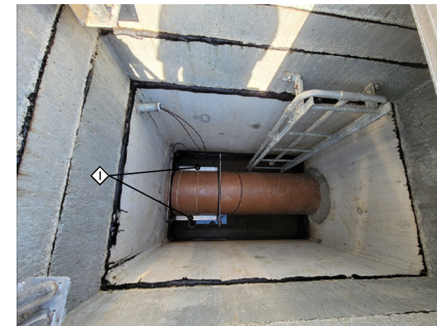
PHOTO: FINAL EFFLUENT FLOWMETER VAULT
