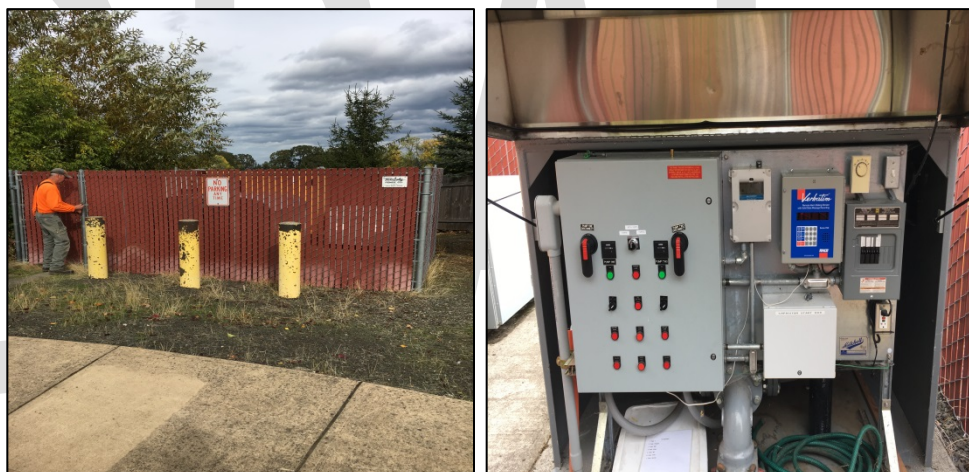
FIGURE 2.3.8 STEELHEAD AND COHO PUMP STATION
