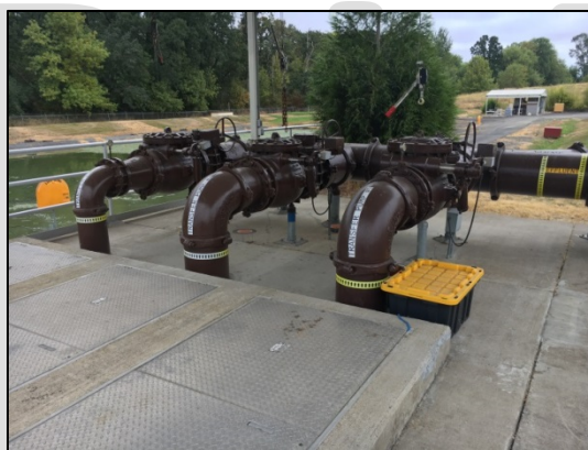
FIGURE 2.3.17 TRANSFER PUMP STATION
