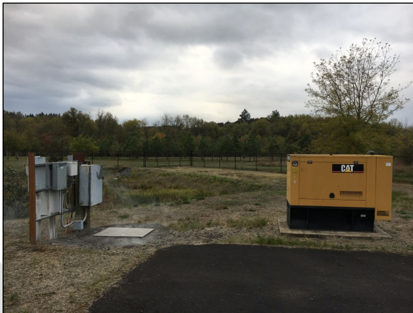
FIGURE 2.3.6 STOWERS PUMP STATION
