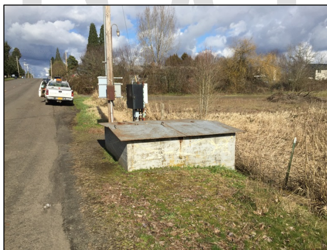
FIGURE 2.3.7 SOUTH MOLALLA PUMP STATION
