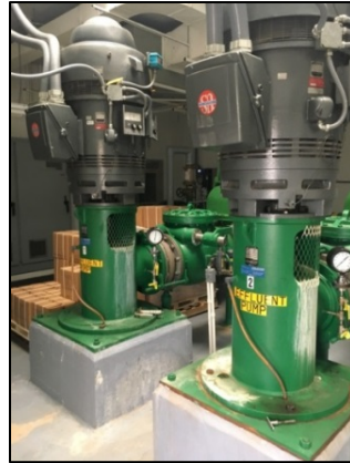
FIGURE 2.3.27 EFFLUENT PUMP STATION
