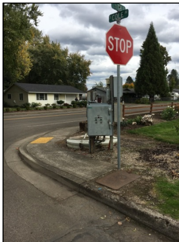
FIGURE 2.3.10 EAST 5 TH AND SOUTH COLE PUMP STATION
