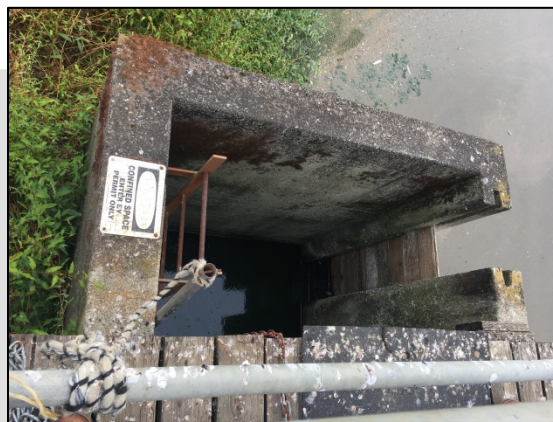
FIGURE 2.3.19 LEVEL CONTROL STRUCTURE
