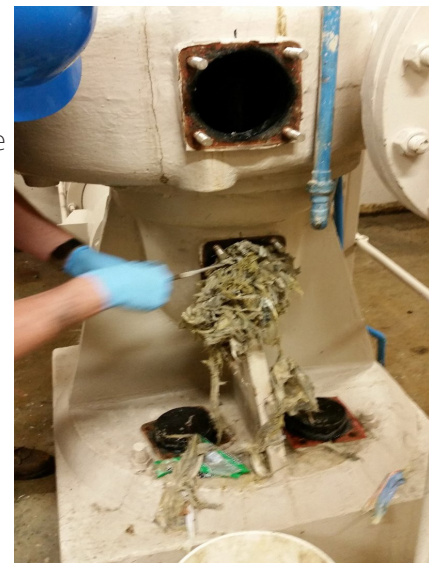
Roseburg Urban Sanitary Authority: There are no easy methods or tools for removing non-flushable wipes from sewage pumps.
