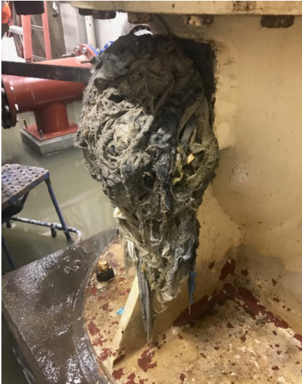
Clackamas Water Environment Services: Wet wipes combined with grease and other non-flushable materials, create ropery mats that clog sewer pumps that workers must remove manually.
