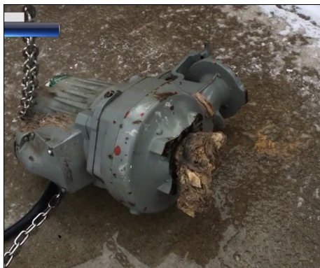
City of Bend: Pumps of All Sizes Clog with Wipes Flushed Down Toilets
